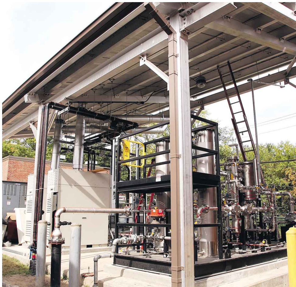
The site where a Water Pollution Control District restaurant grease-receiving station could be built.
