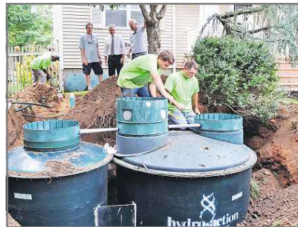
An advanced septic system is installed at a Nesconset home in 2015.
