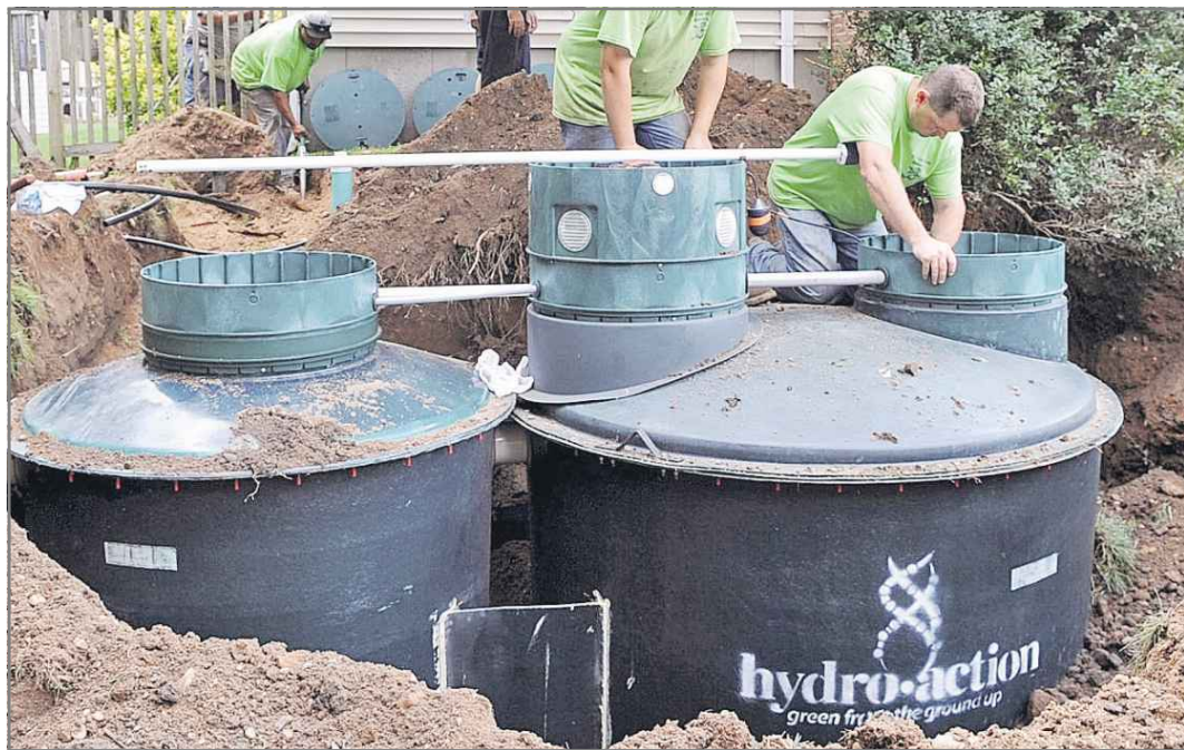
Workers install a septic tank in Nesconset. A plan in Suffolk would ease cesspool replacement.
