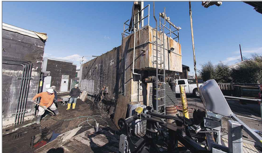
Construction on Ocean Beach's sewer treatment plant, shown Monday, will nearly double its efficiency.
