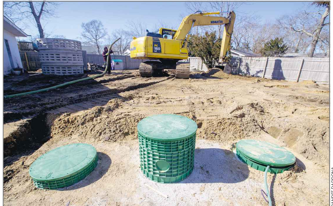
An advanced septic system that removes nitrogen from water being installed at a home last year.
